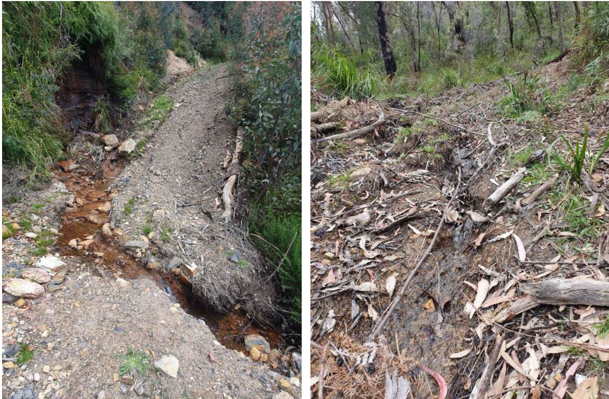
Plate 1 Examples of rill erosion and moving water present on existing track
