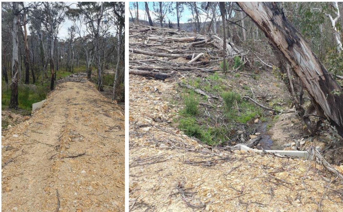
Plate 2 Existing culverts to the south of the study area, with moving water and growth in the channels
