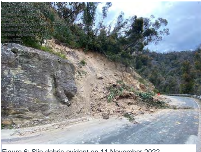
Figure 6: Slip debris evident on 11 November 2022
