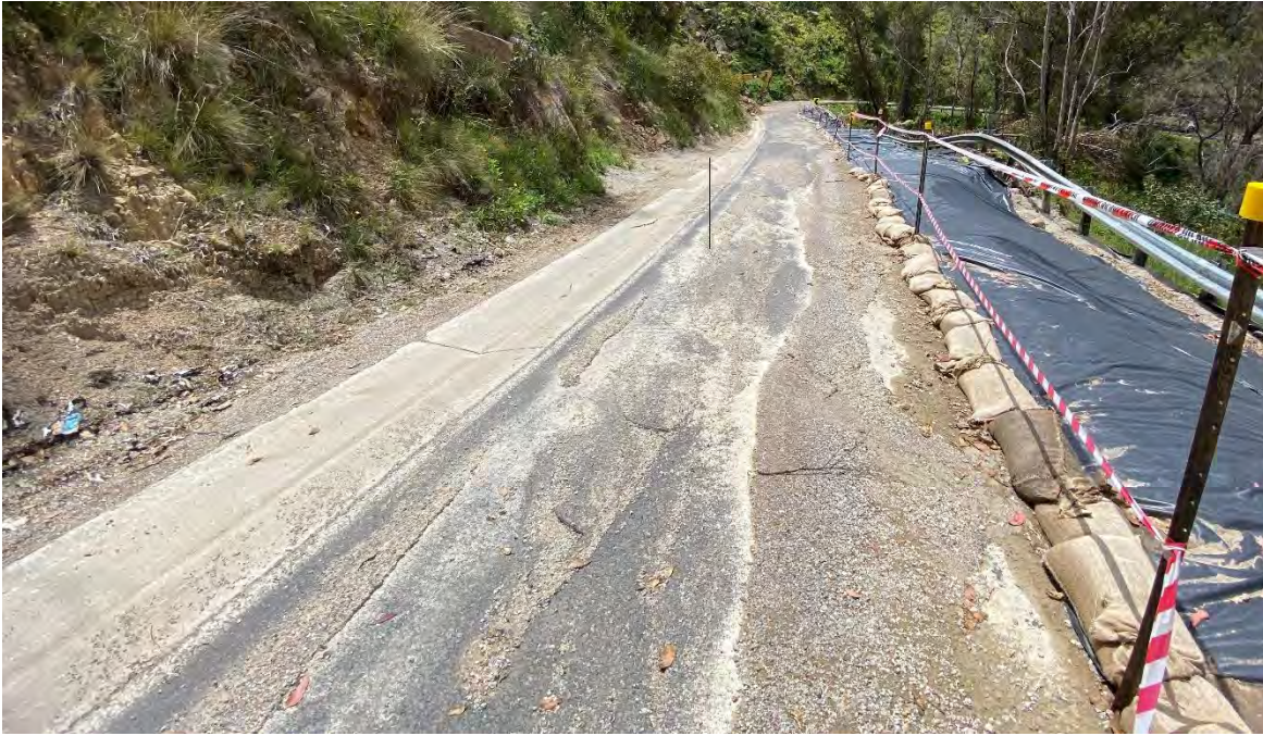
Figure 5: Loss of downslope lane - 2022
