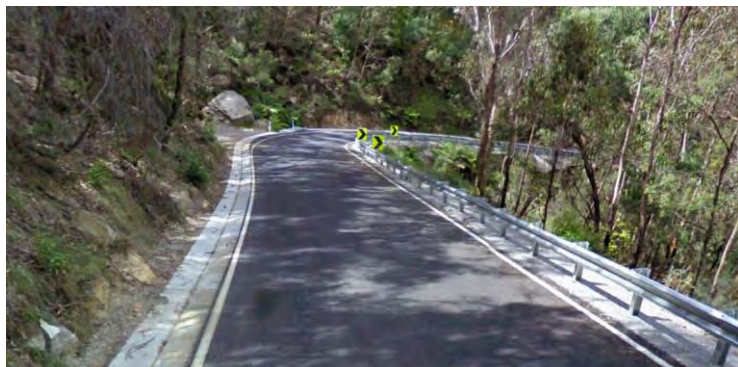
Figure 3: Section of Wolgan Road subject to instability (image dated February 2010; prior to current instability)
