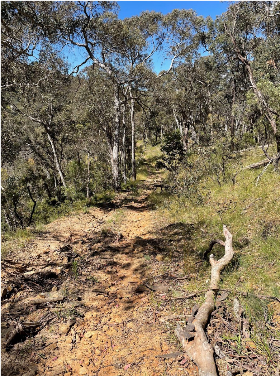
Plate 4.8 Proposed drill pad location MB2206 located across the existing access track. Soil deposits are extensively rutted by slope wash
