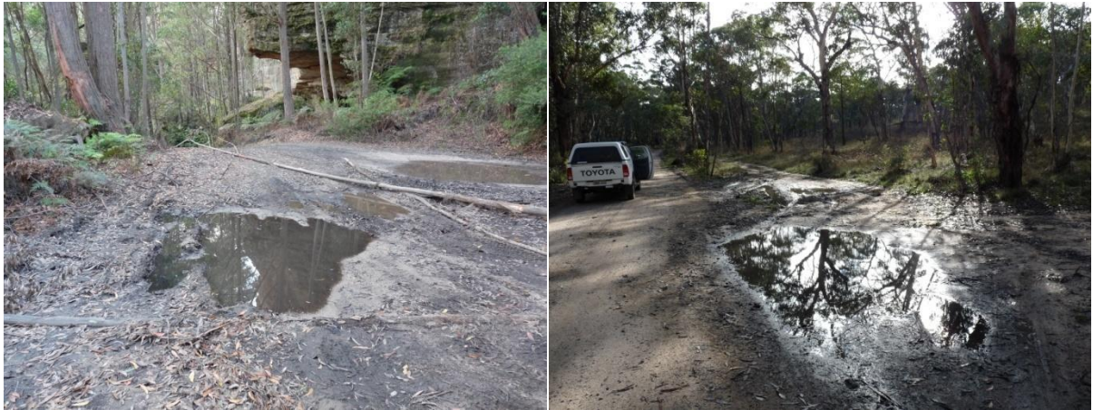
Plate 8: Water pooling in wheel ruts that have been formed by 4WD use of the study site
