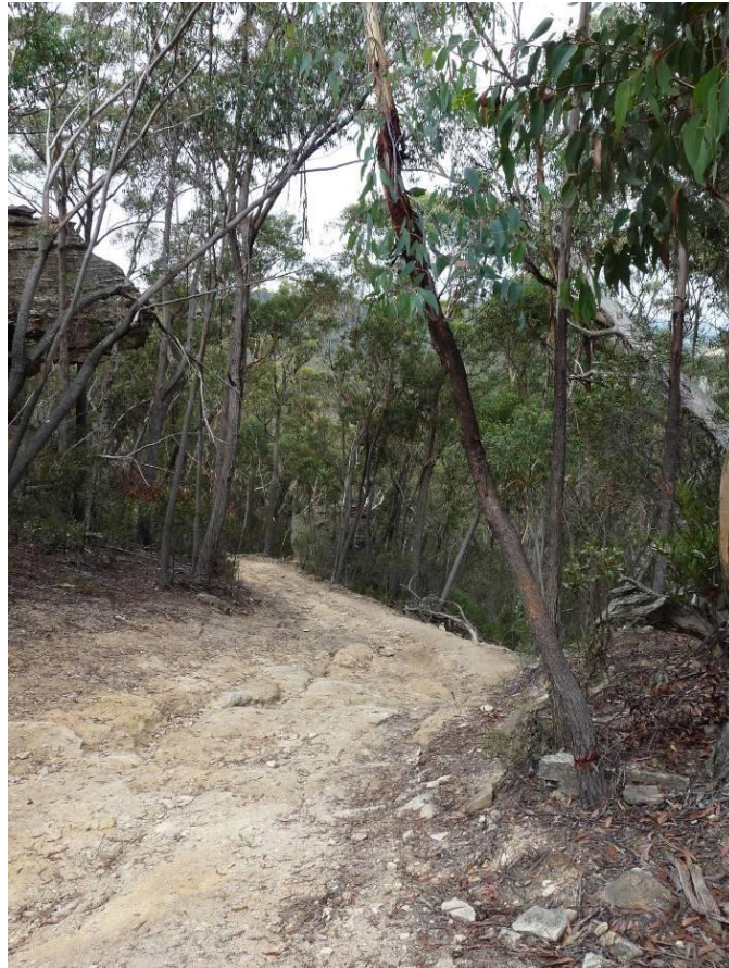
Plate 3: Severe erosion on Bicentennial National Trail leading to the Blackfellows Hands Reserve, within the Ben Bullen State Forest.
