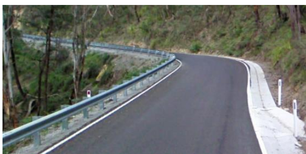
Figure 3-1 – Flexible Safety Barriers (Wolgan Road)
