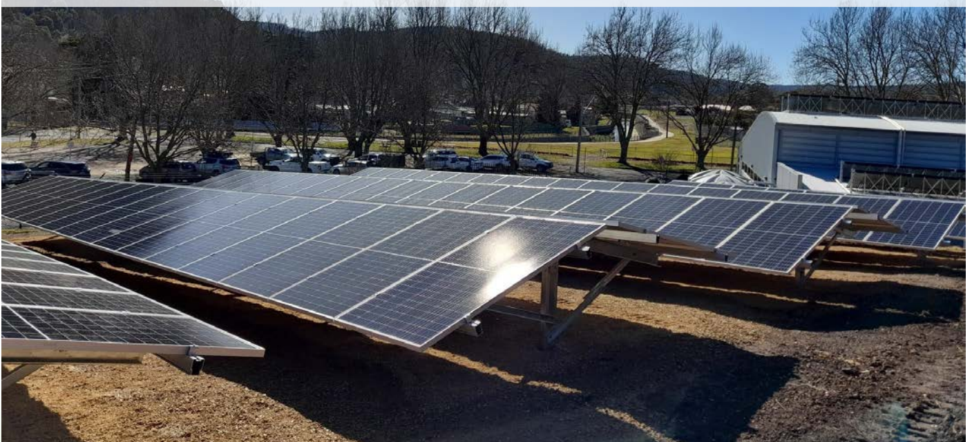
JM ROBSON AQUATIC CENTRE SOLAR PANELS
