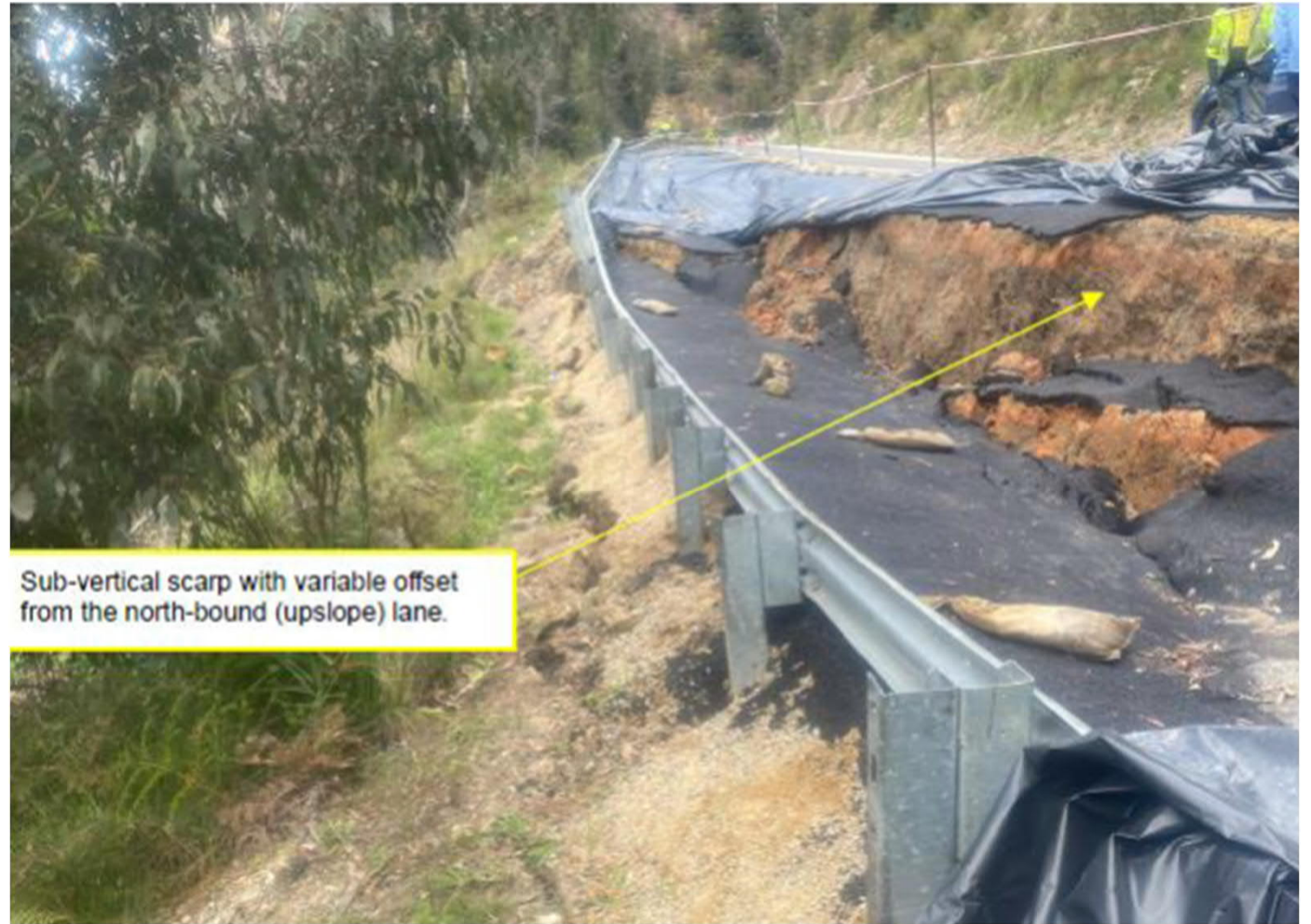
Figure 5: Looking south at Hazard 2B, photograph taken 10 th October 2022
