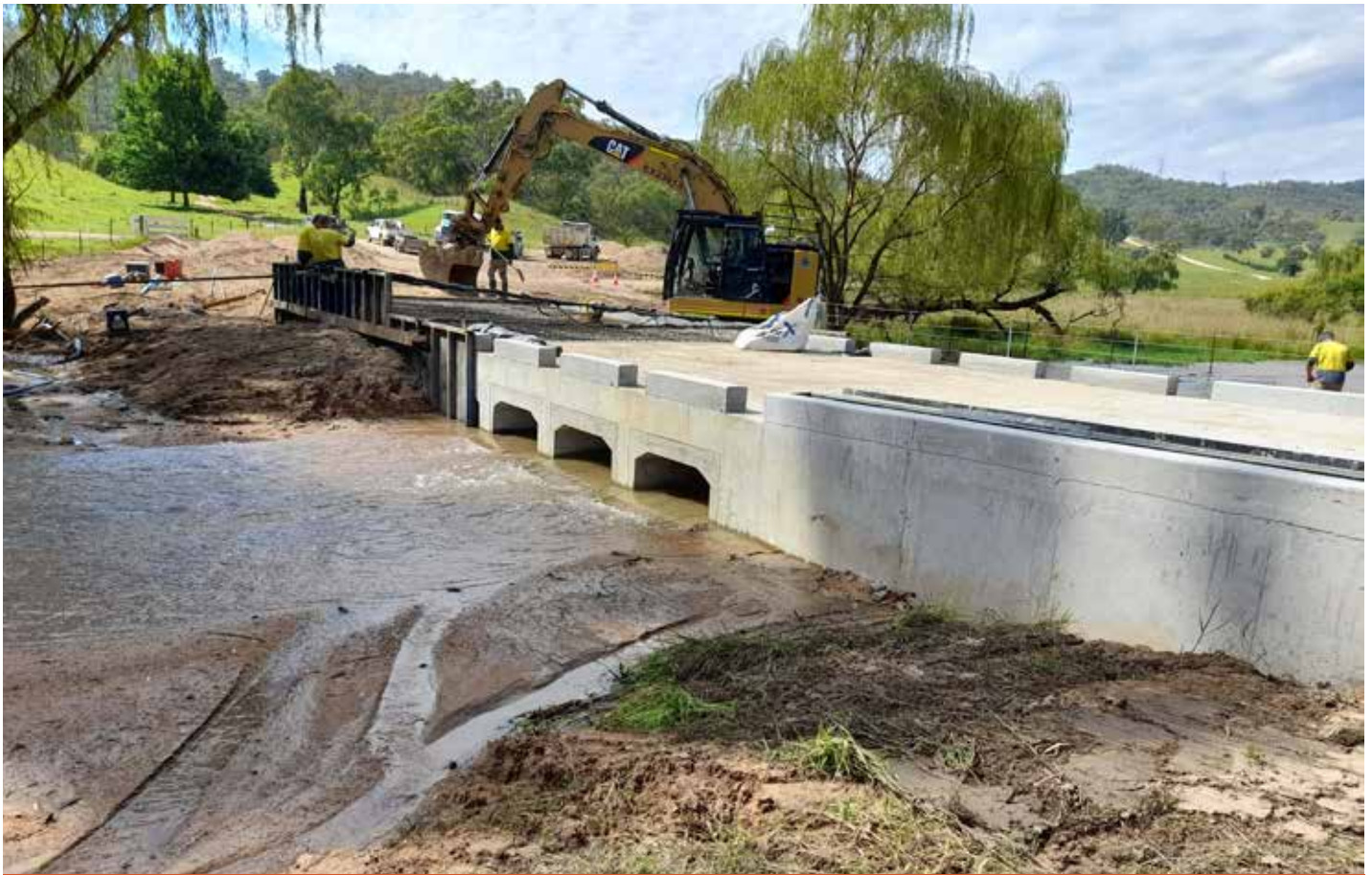
Cullenbenbong Causeway - reconstruction has provided the opportunity to improve the resilience of local assets in the wake of these disasters.
