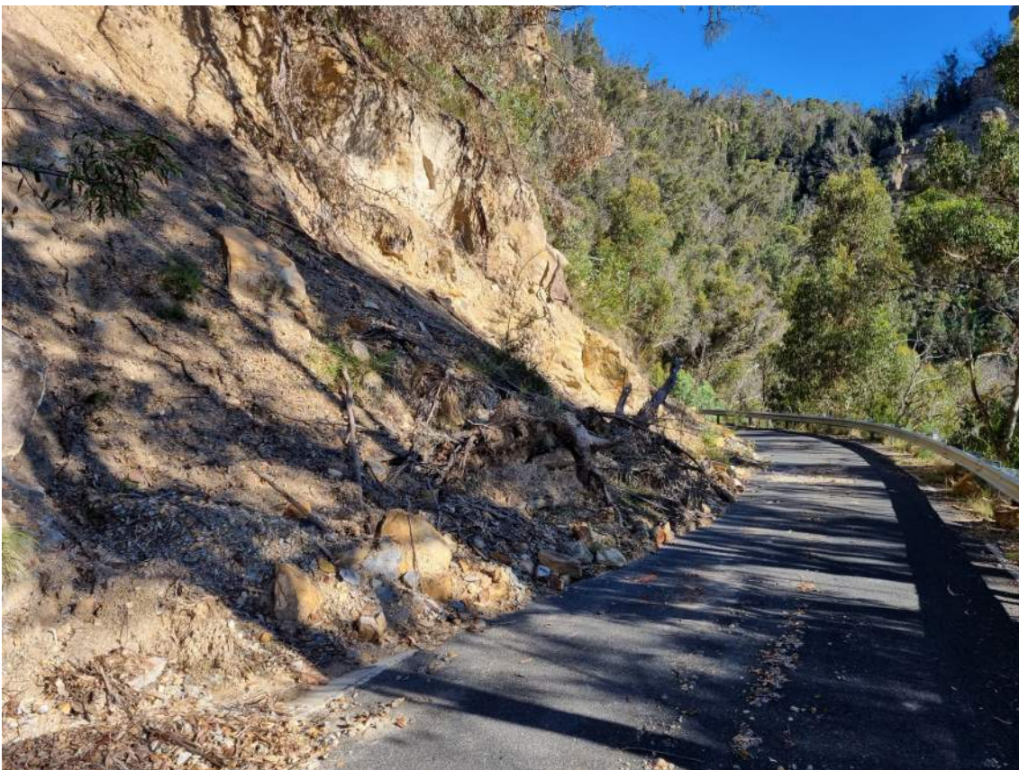
Figure 4 Upslope batter failure in colluvium, talus and weathered rock.
