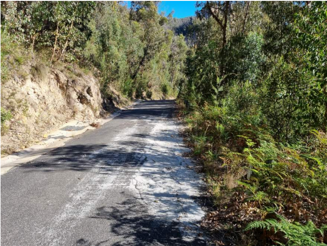
Figure 3 Localised tension cracking in downslope lane.
