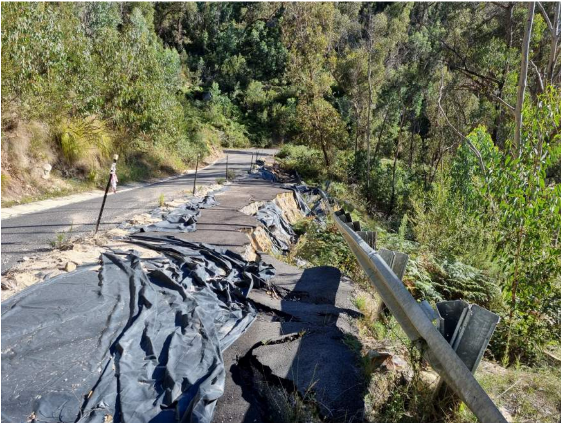
Figure 5 Embankment failure comprising slumping of fill materials below downslope lane. Upslope lane remains trafficable.
