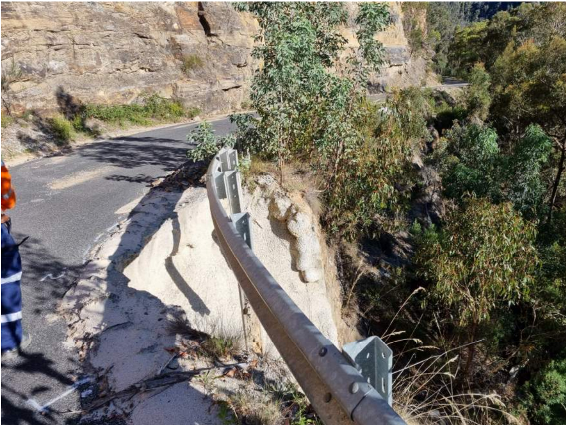
Figure 2 Localised failure of drystone wall.
