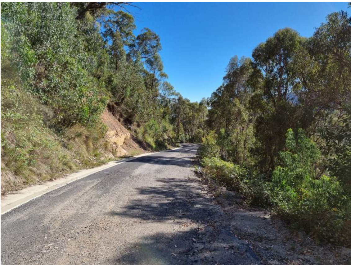
Figure 6 Example of lower section of Wolgan Road in apparent good condition. Asphalt and subbase removed for reuse on Donkey Steps track.
