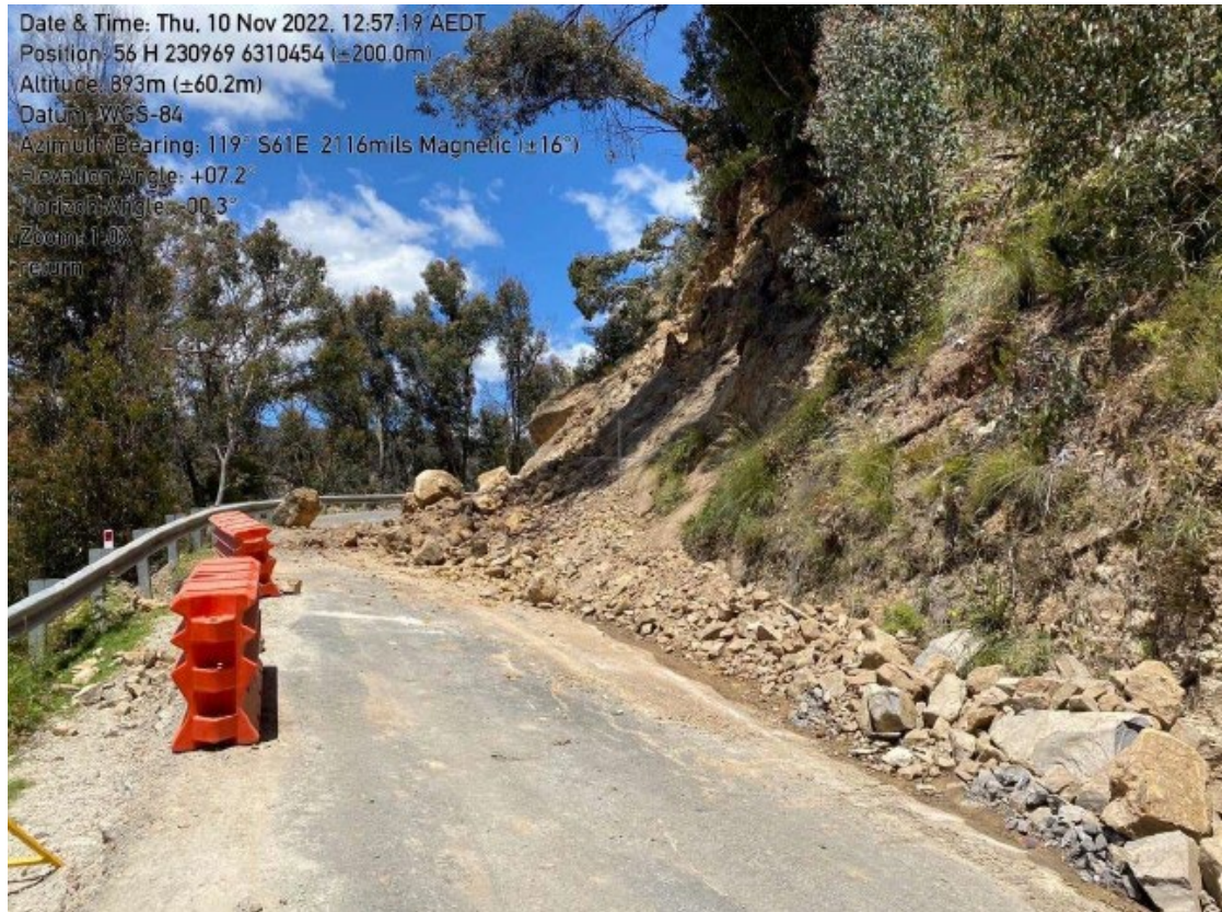
Event 85 - Aerial photogrammetry showing landslide, captured 15/11/2022.
