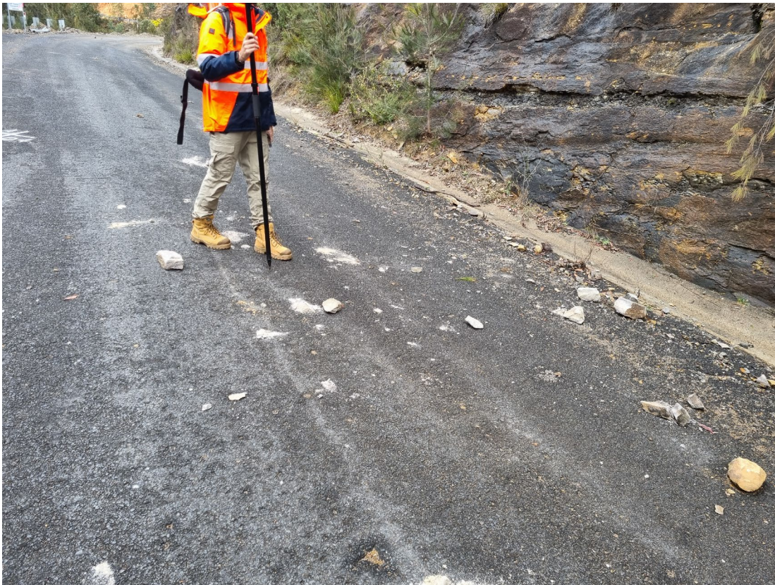
Figure 10 Extremely small rockfall fragments on road below cliff in Domain 1.
