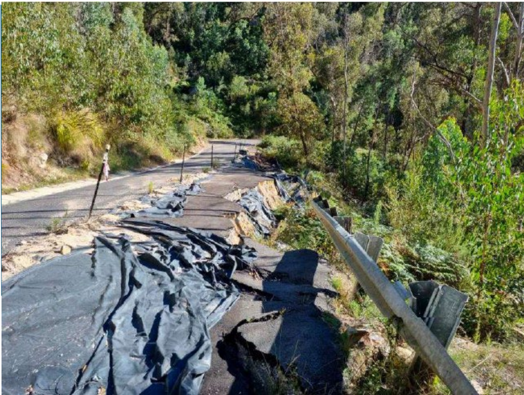
Event 73 - Photo from GHD report showing embankment failure, taken 18/02/2025.
