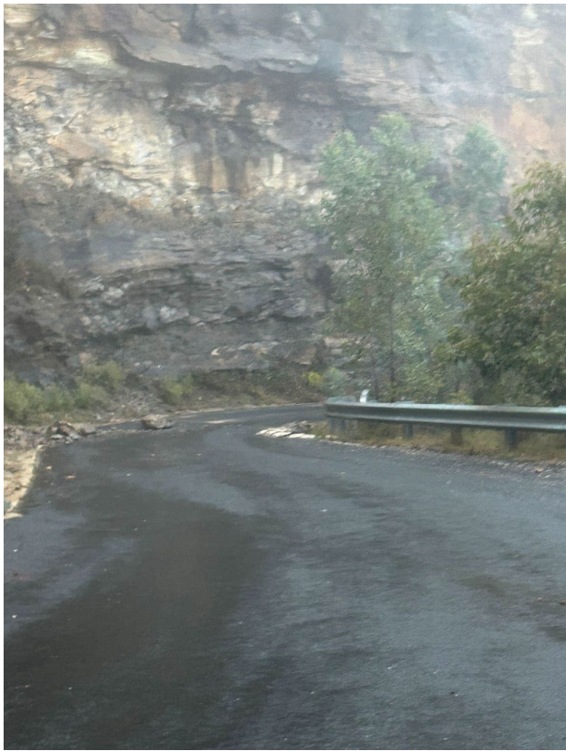
Event 91 - Resident's photo of rockfall, taken post road closure (11/2025), exact date unknown.
