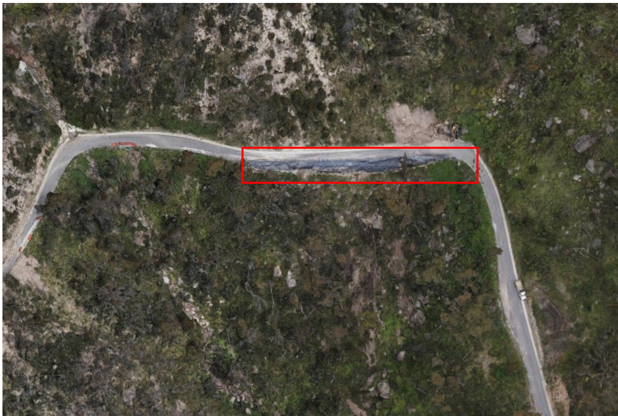
Event 73 - Aerial photogrammetry showing embankment failure, captured 29/08/2022.
