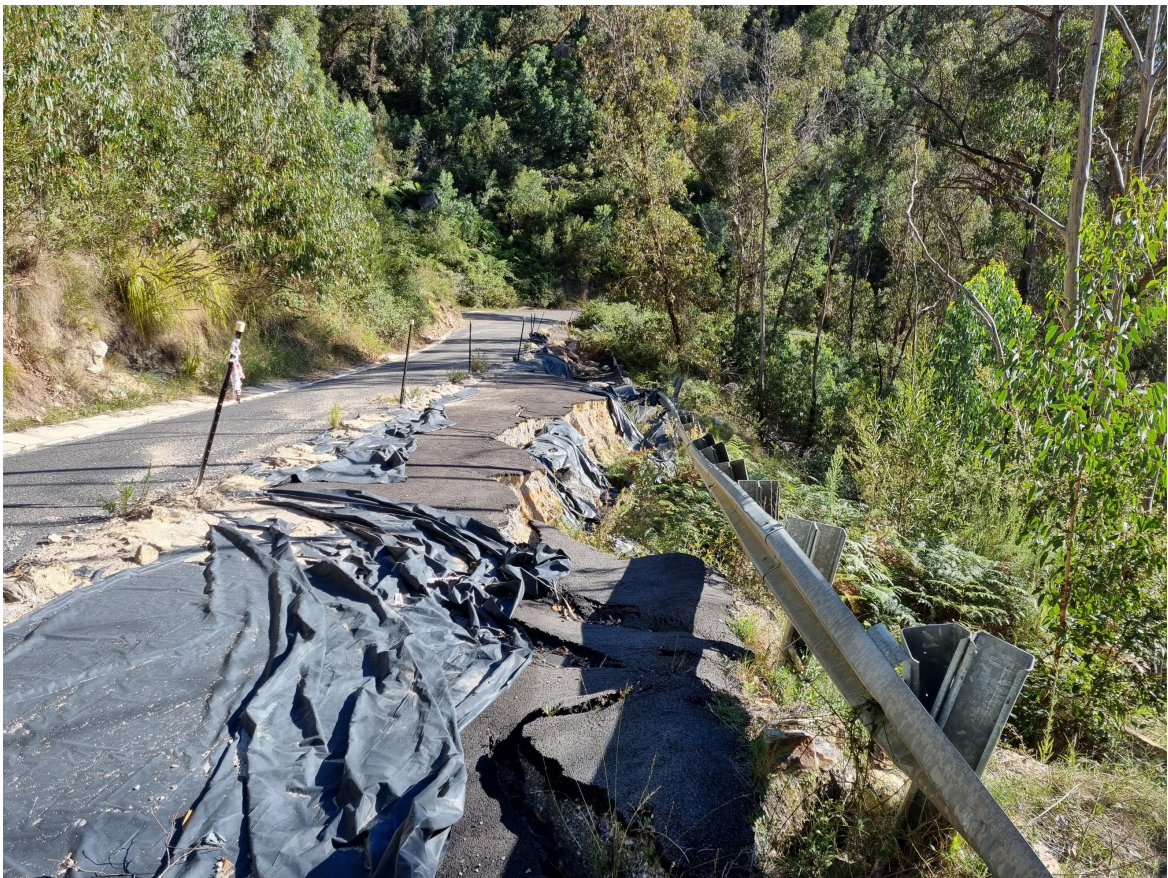
Figure 17 Embankment slide comprising slumping of fill materials below downslope lane. Upslope lane remains trafficable.
