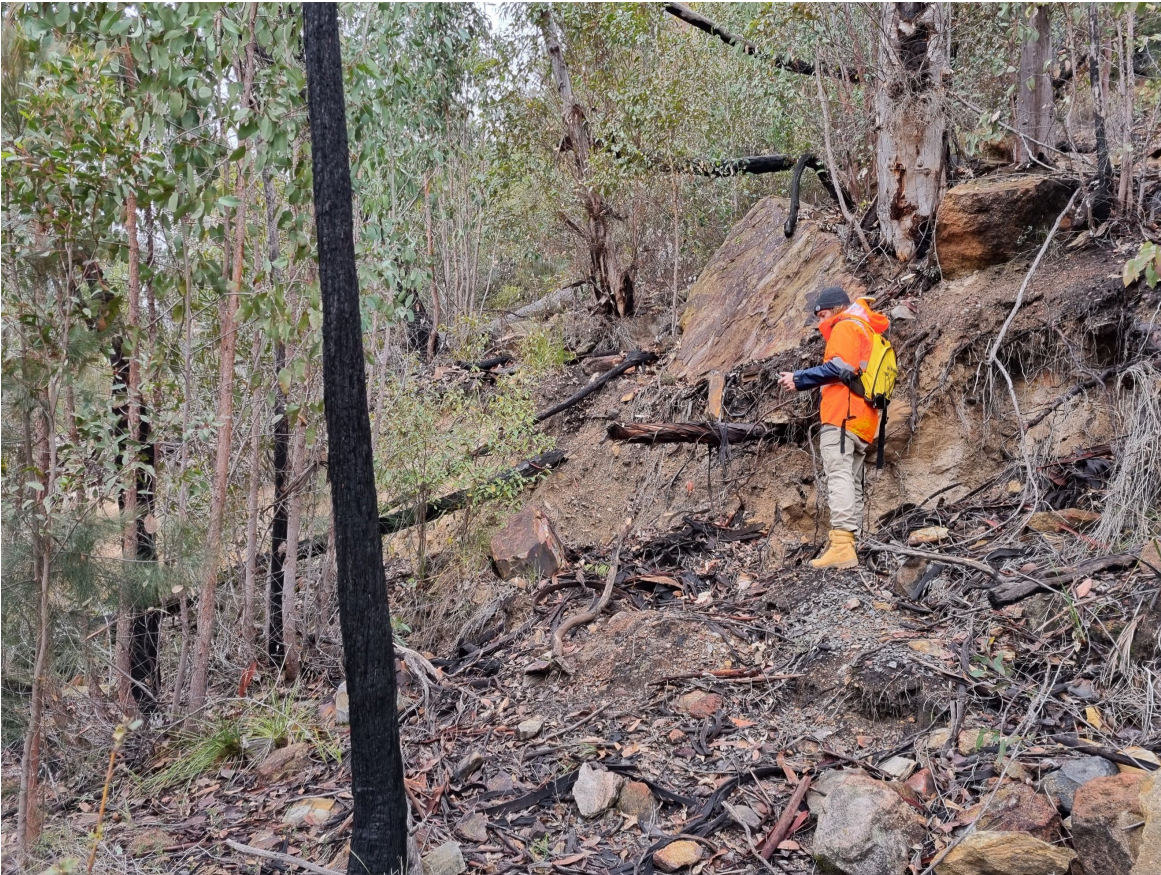
Figure 13 Landslide crown / head scarp on colluvial slope above road.
