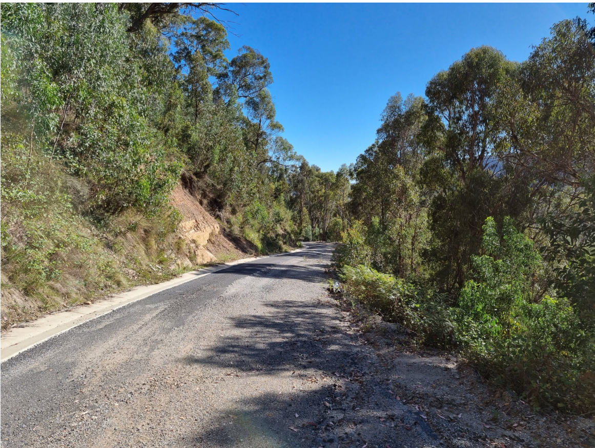
Figure 20 Example of lower section of Wolgan Road in apparent good condition. Asphalt and subbase removed for reuse on Donkey Steps track.
