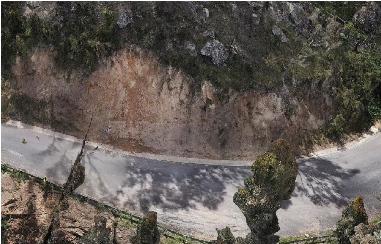
Event 84 - Aerial photogrammetry showing landslide, captured 15/11/2022.
