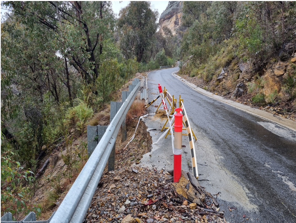
Figure 15 Shallow downslope road shoulder failure.
