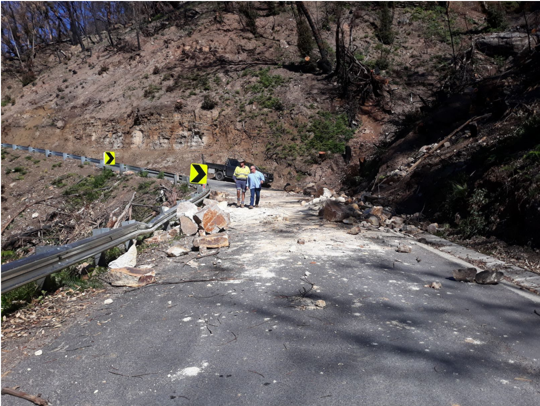
Event 59 - Council photos of rockfall debris, taken around 11/08/2020.
