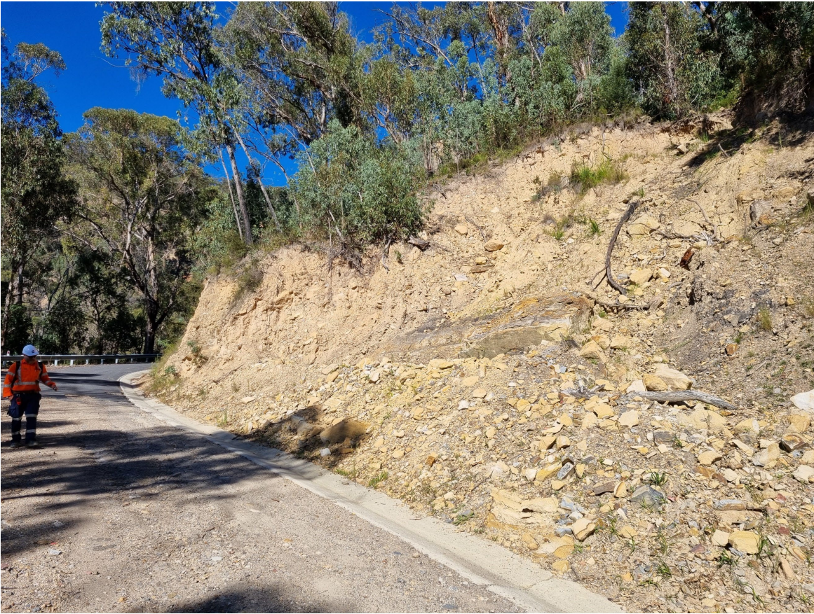
Figure 19 Example of upslope batter failure in colluvium, talus and weathered bedrock
