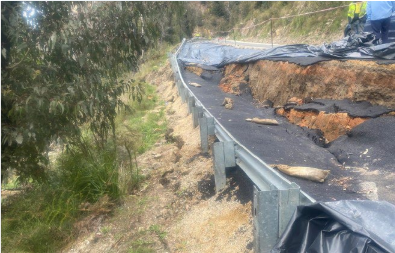
Event 73 - Photo from Golder report showing embankment failure, taken 10/10/2022.
