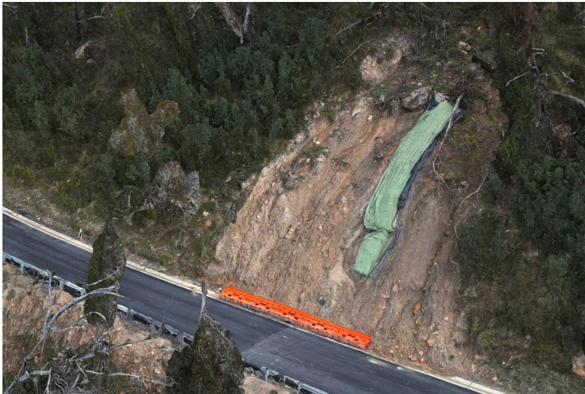
Event 74 - Aerial photogrammetry showing landslide, captured on 29/08/2022.
