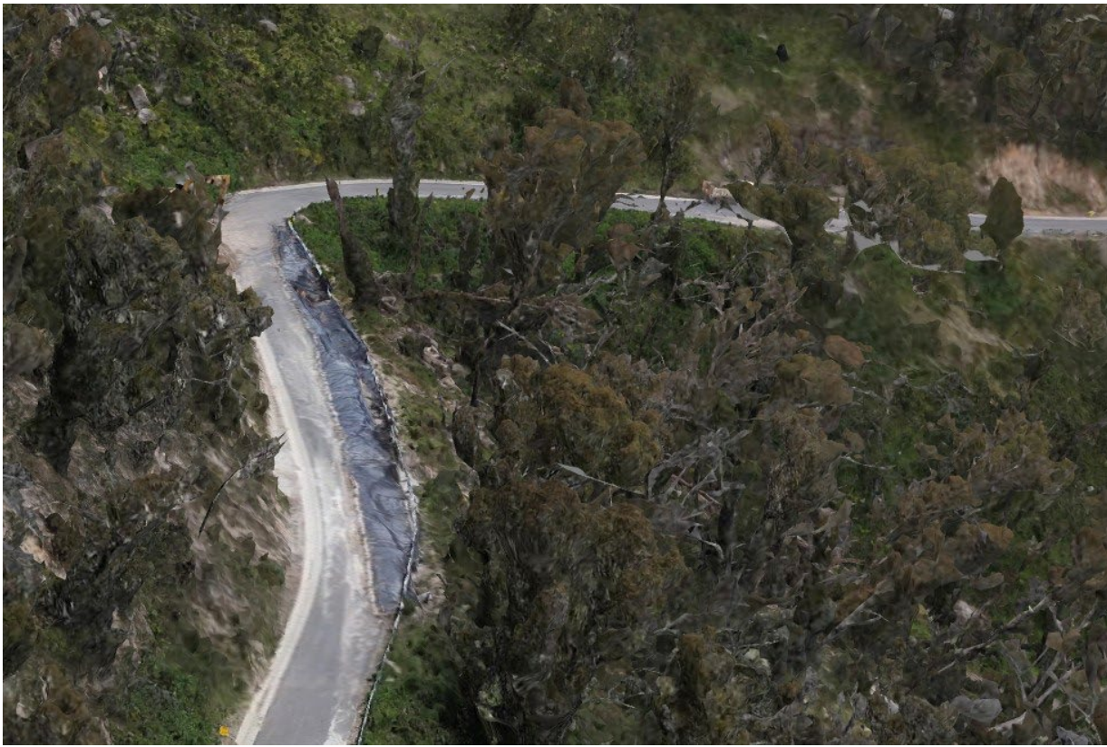
Event 73 - Aerial photogrammetry showing embankment failure, captured 29/08/2022
