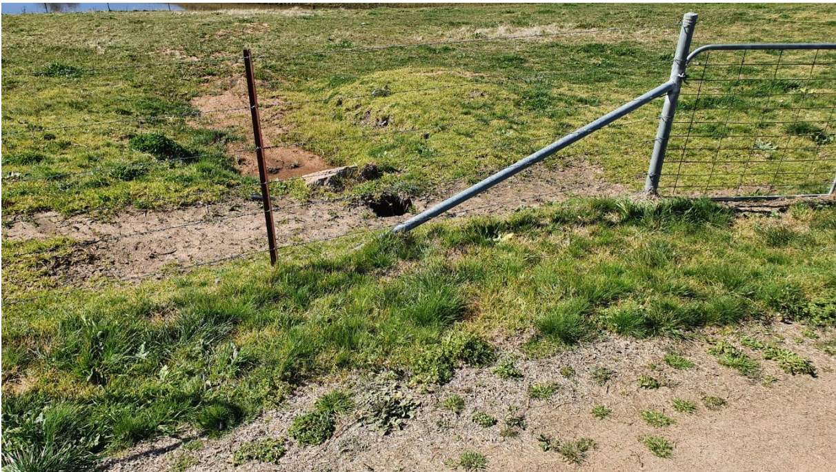
Approximate Ch 1620 looking East at tunneling behind culvert stone headwall in property. Stable verge.
