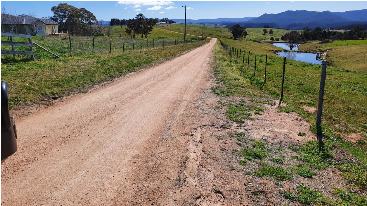
Approximate Ch 1240 looking North at good road shape and condition. Stable verges and drainage.
