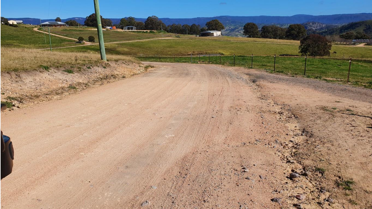
Approximate Ch 700 looking West at minor erosion.
