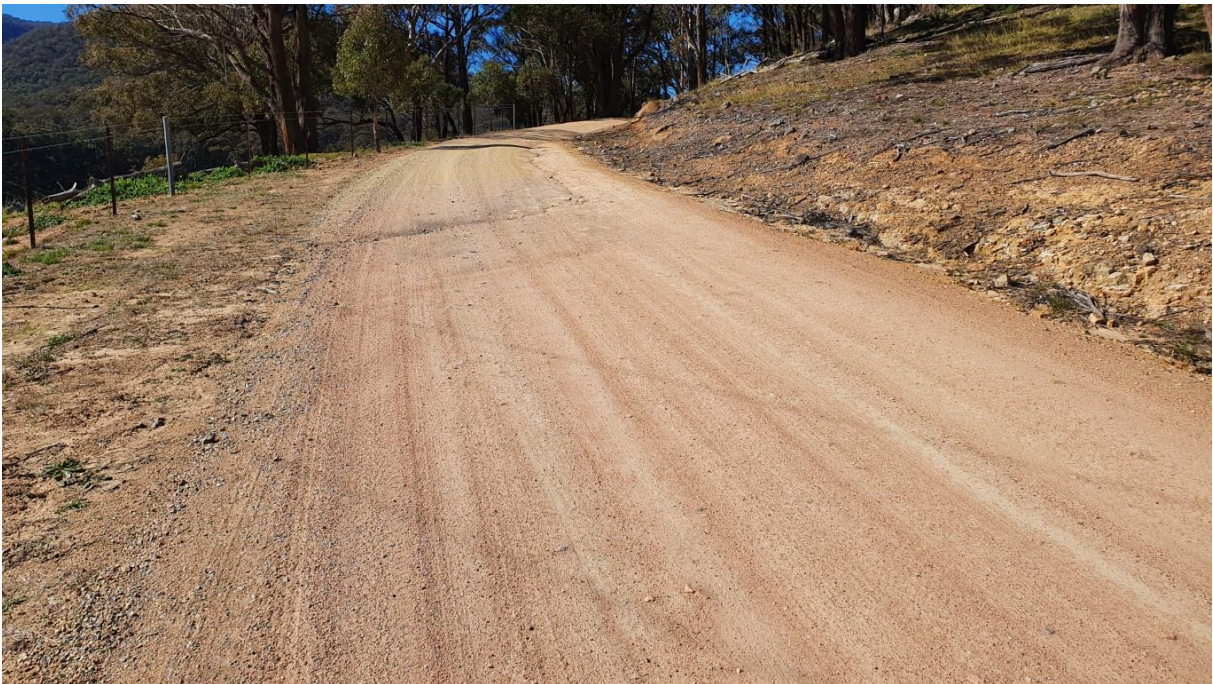
Approximate Ch 700 looking East at minor erosion.
