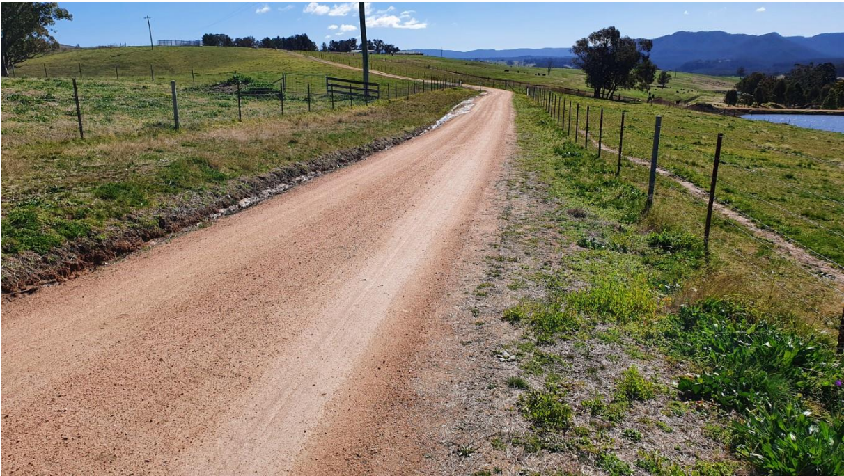
Approximate Ch 1500 looking North at minor drainage scour LHS. Good road shape & condition, stable verges.
