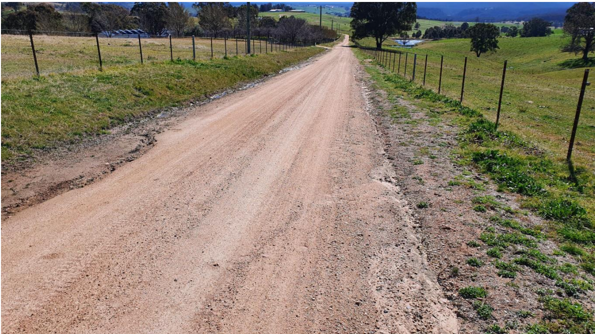
Approximate Ch 1120 looking North at minor erosion and drainage shaping required. Stable verges and runoff.
