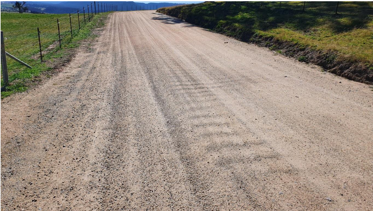
Approximate Ch 830 looking Northeast at minor corrugations. Stable verges.
