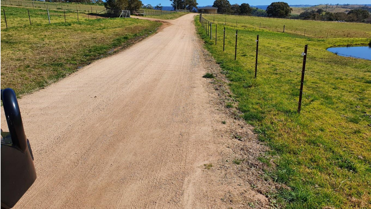
Approximate Ch 900 looking Northwest at minor corrugations and drainage shaping required. Stable verges and runoff.
