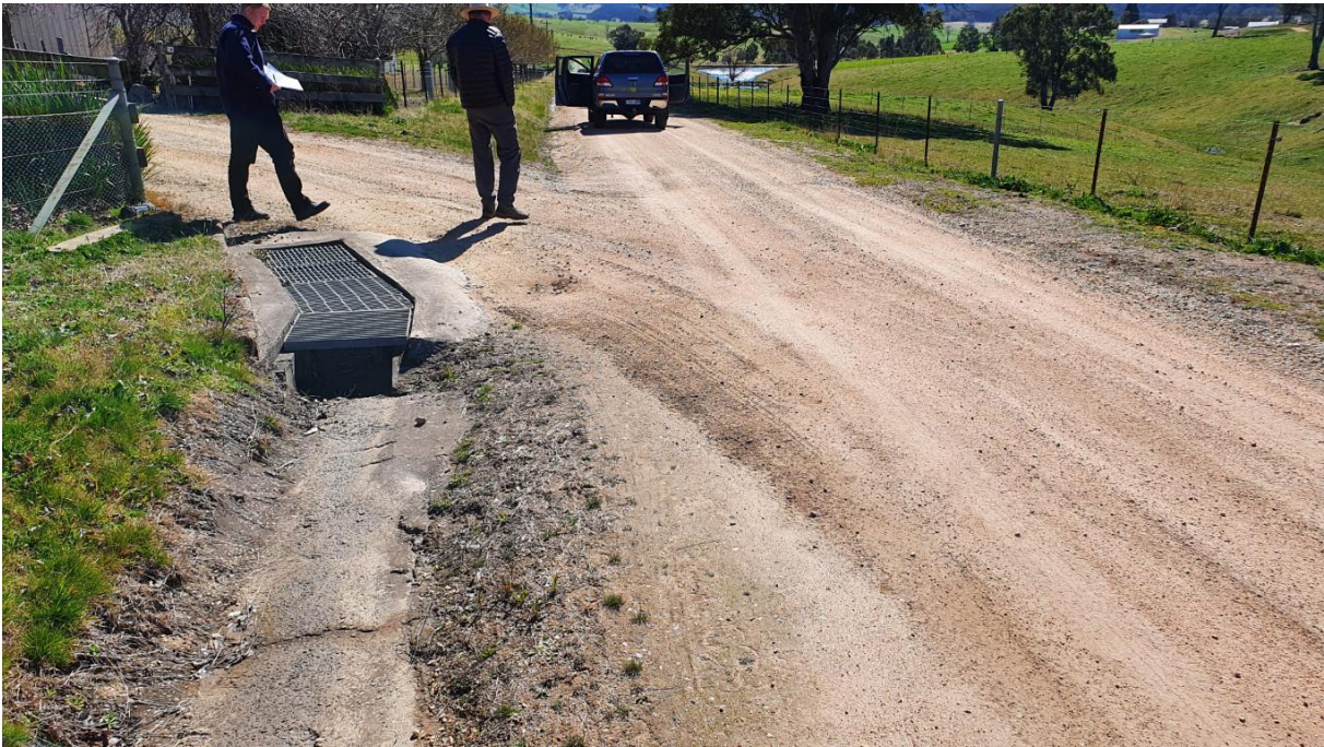
Approximate Ch 1200 looking North at very good stable drainage, road and verge areas.
