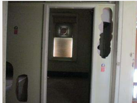
Plate 143: Interior showing damage to walls.
