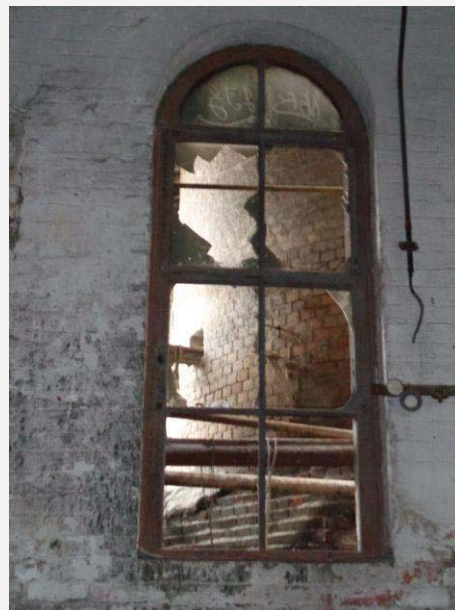
Plate 21: Broken and missing glazing.
