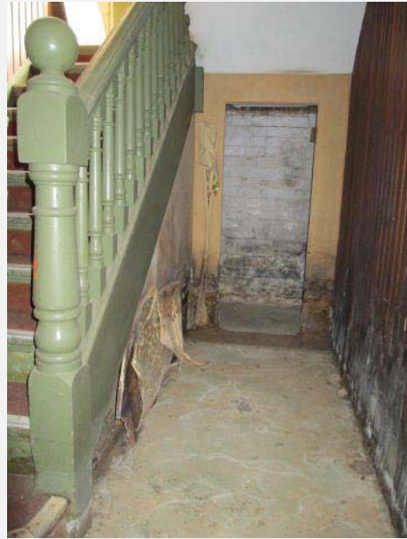
Plate 152: Interior to basement showing unsympathetic wall finish (timber panelling, right) and brick infill and damage to walls.
