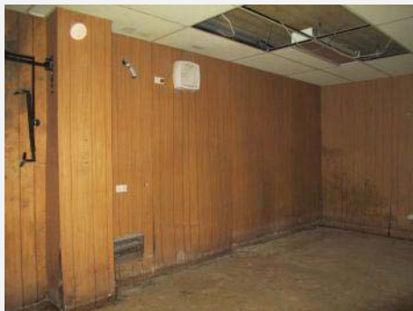
Plate 148: Interior showing unsympathetic additions, timber panelled walls, ceiling grid and electrical services. Note: Evidence of mould on walls.
