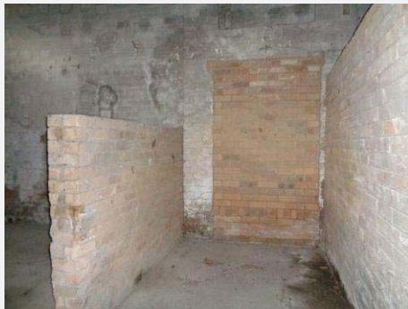
Plate 30: Machinery room showing unsympathetic brick wall additions and infills.
