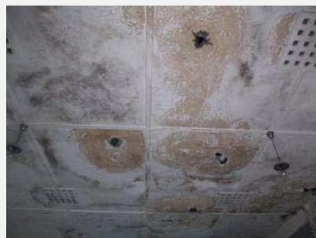
Plate 201: Interior showing water damage to ceilings.
