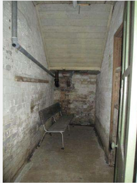
Plate 153: Interior to basement level under stairway showing timber panelling to stair and evidence of mould on walls.
