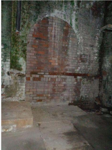
Plate 28: Machinery room showing unsympathetic brick infill to archway and severe moisture issues to west wall.
