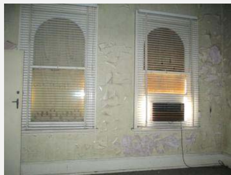
Plate 141: Interior showing paint peeling on walls, unsympathetic air conditioning unit addition.
