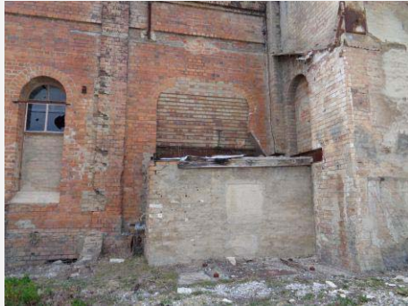
Plate 10: Detail area of west elevation showing damage to brickwork, infilled openings, brick plinth and broken glazing.
