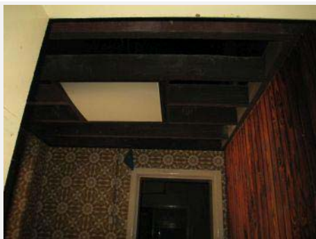
Plate 144: Interior showing missing ceiling, unsympathetic wall finish including timber panelling.
