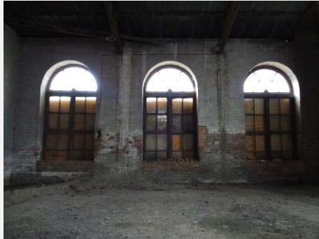
Plate 34: Eastern room showing damage to brickwork, timber framed windows and rubble floor.
