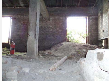
Plate 231: Interior room (south east) showing absent floor and rubble.
