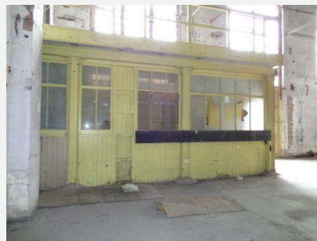
Plate 23: Switchboard room showing painted timber panelling and glass panels.
