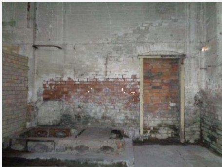
Plate 32: Machinery room showing unsympathetic brick wall infills in doorway.
