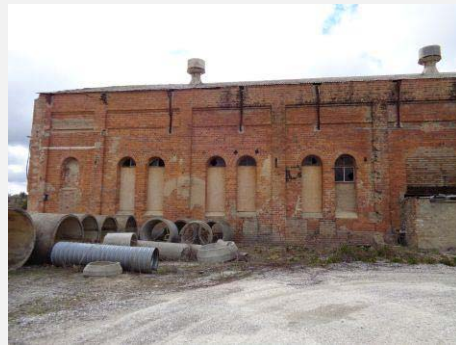
Plate 5: Part west elevation showing original building with some discolouration on brickwork caused by moss.
