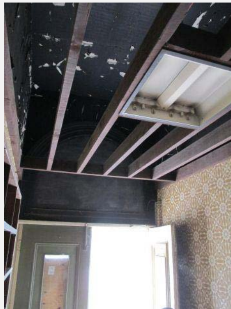
Plate 137: Interior showing ceiling at south entrance and missing ceiling, unsympathetic wall finish.
