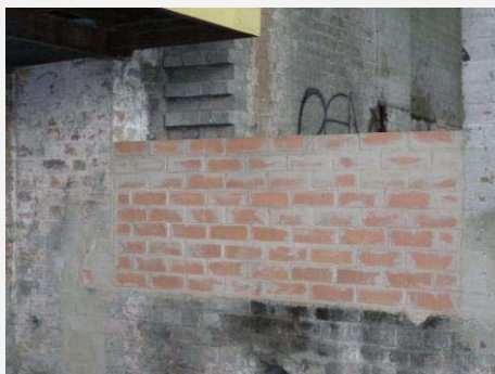
Plate 22: Machinery room (located south west) shows unsympathetic infill brickwork.
