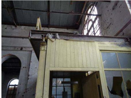
Plate 24: Switchboard room showing steel frame floor above and broken glazing.
