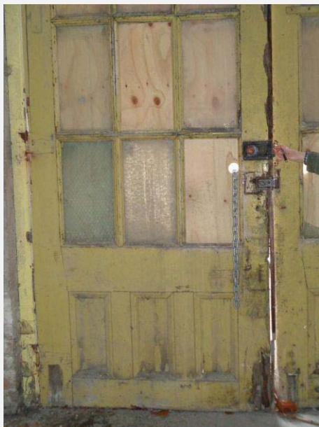
Plate 26: Entry door to south elevation showing missing glazing panels and damage to timber door.
