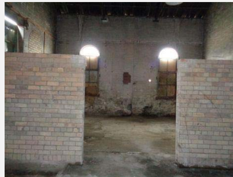
Plate 31: Machinery room showing unsympathetic brick wall additions.
