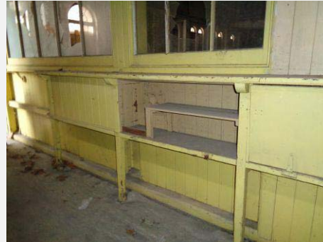
Plate 25: Switchboard room showing timber joinery.
