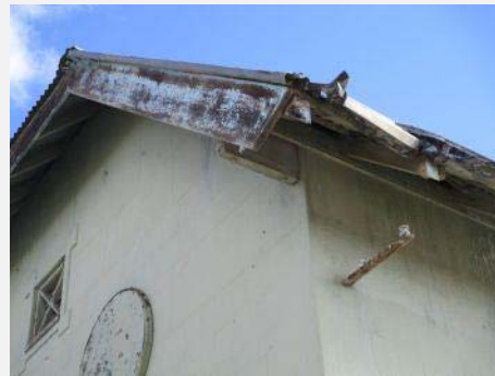
Plate 209: Detail at north west corner of roof showing damage to gutters and timber roof trims.
