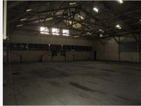
Plate 203: Interior of main room showing water damage to floor boards.
