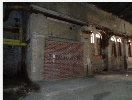
Plate 17: Interior eastern wall showing unsympathetic infill brickwork.
