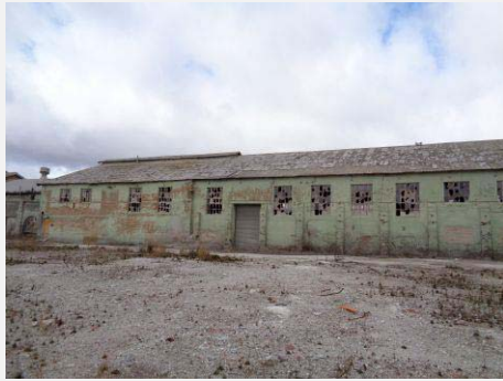
Plate 49: Boilerhouse north elevation showing roof, walls and windows in poor condition.
