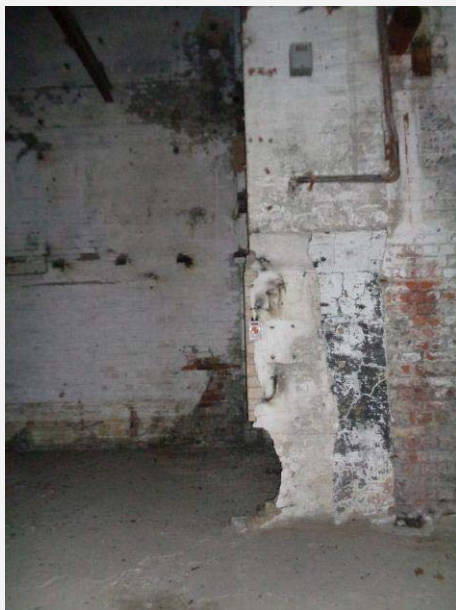
Plate 20: Broken and missing brickwork on column.
