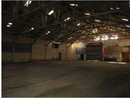
Plate 202: Interior of main room showing water damage to floor boards.
