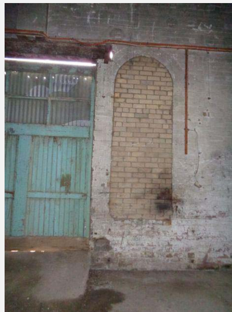
Plate 27: Machinery room showing unsympathetic brick infill to window opening, timber service door with concrete ramp.
