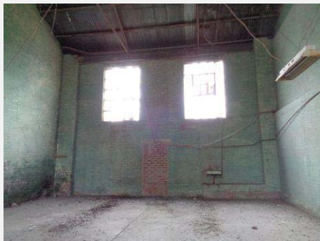
Plate 65: Interior of Central room showing unsympathetic brick infill to opening in north wall.
