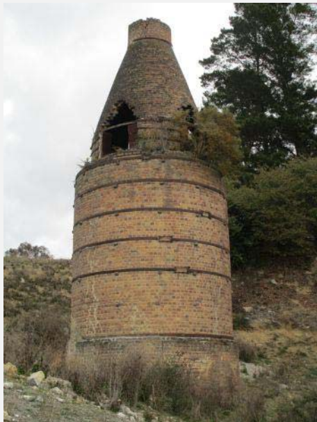
Plate 234: Brick Bottle Kiln (south) showing broken and missing bricks and weed growth.
