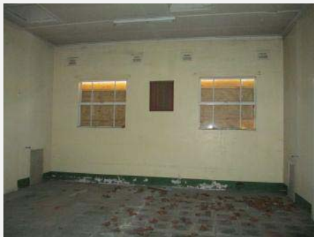
Plate 128: Interior showing room to east end with damage to linoleum floor finish.
