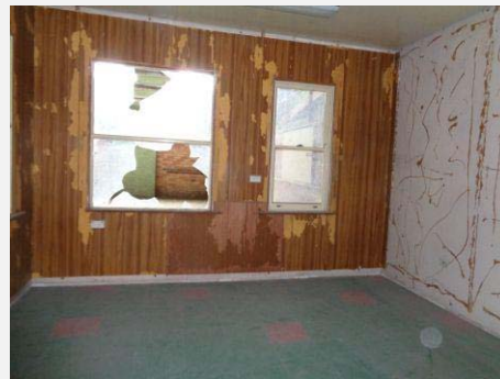
Plate 70: Interior of Eastern room showing unsympathetic addition with timber panelling to walls.
