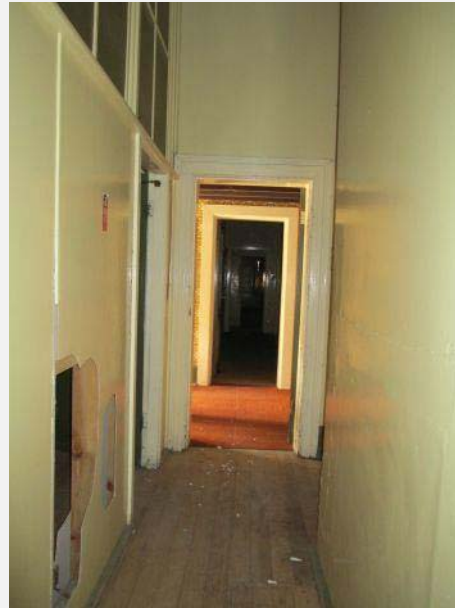
Plate 147: Interior showing damage to walls and stripped floor finish. Unsympathetic addition beyond (carpet finish).
