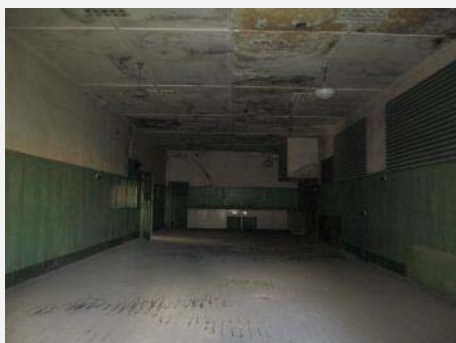
Plate 200: Interior showing water damage to floors and ceilings.
