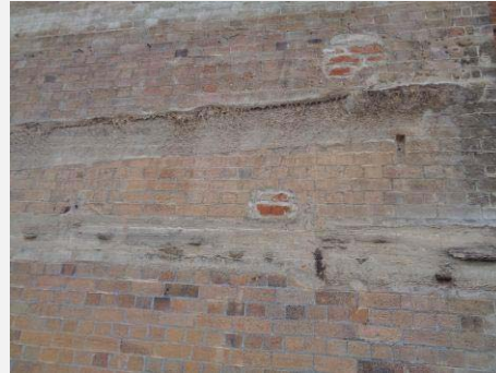
Plate 11: Detail area of west elevation showing unsympathetic patchwork to bricks.
