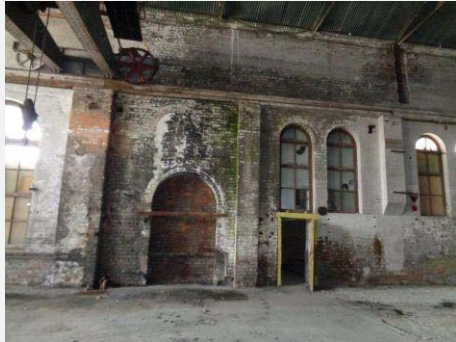
Plate 18: Interior looking east showing infill brickwork to opening, presence of moss on walls.
