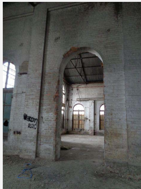
Plate 37: Eastern room showing damage to brick openings.
