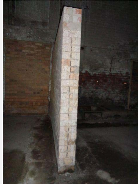
Plate 29: Machinery room showing unsympathetic brick wall additions and moisture issue to floor.
