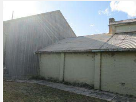
Plate 186: Part south elevation showing water ingress.
