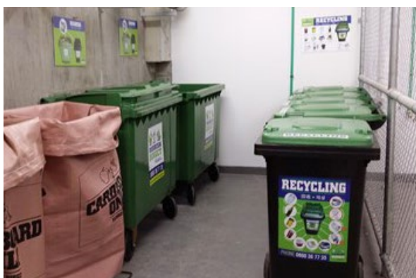
Figure 3-145 Waste and recycling areas should allow for sufficient space to manoeuvre bins and sort waste for recycling
