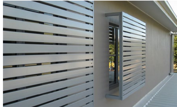
Figure 3-99 Poorly executed privacy screens. These block outlook, sunlight and daylight to windows and reduce amenity of room.
