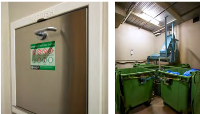
Figure 4W.6 For taller developments, garbage chutes can be located on floors to allow for convenient disposal of waste and recycling
